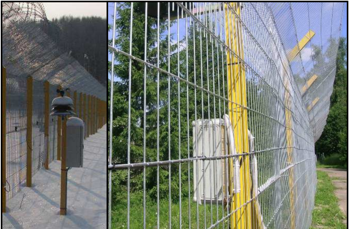
Figure 4. FU-16 (on additional post).
